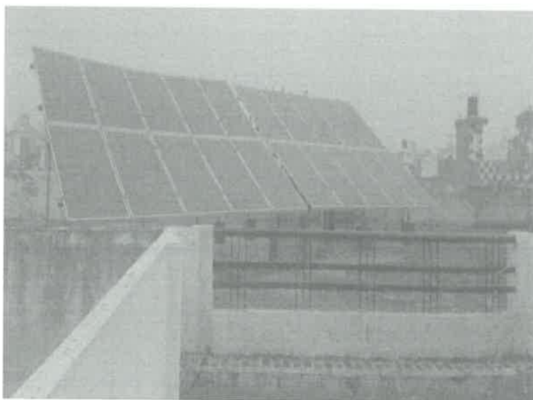
Solar Power Plant in the College
