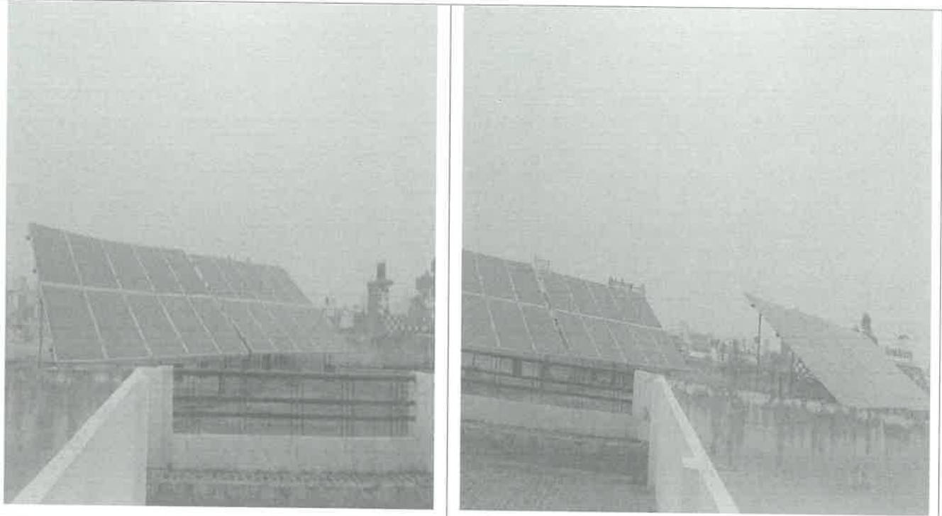
Solar Power Plant in the College
