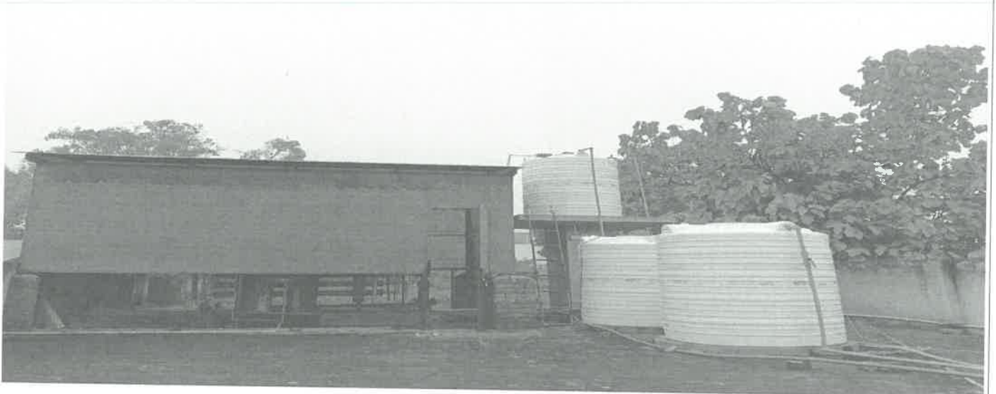
Centralised R. O. Plant in the College
